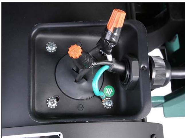
Figure 84. G0605X motor junction box.
